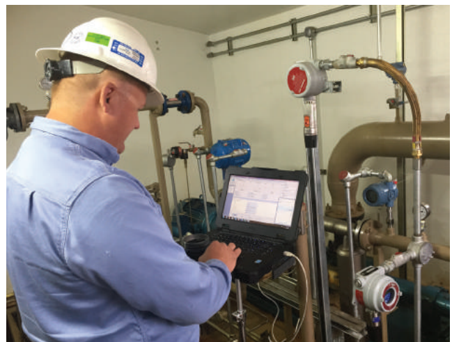
A service technician performs meter verification.
