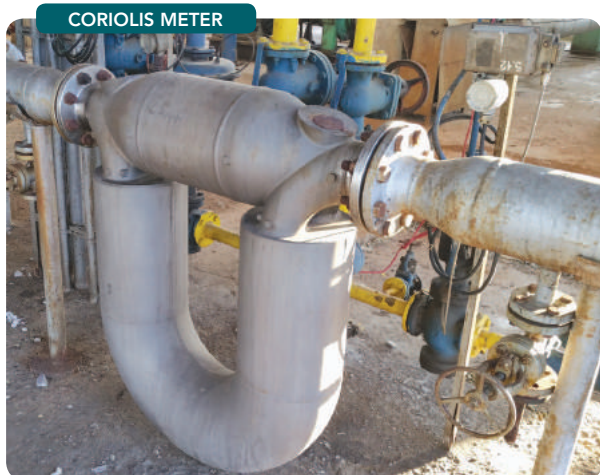
Figure 1. This flow meter has enabled a better mass balance, leading to significant improvement in plant efficiency.
