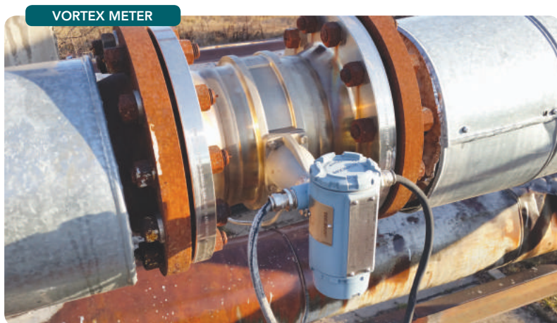
Figure 2. The meter decreased steam leaks dramatically, increasing steam system efficiency and providing very fast payback.
